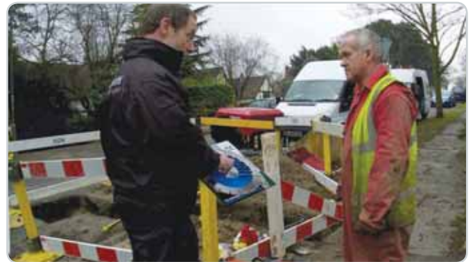
Service & support on site
